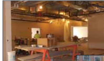
Interior of ventilator unit
